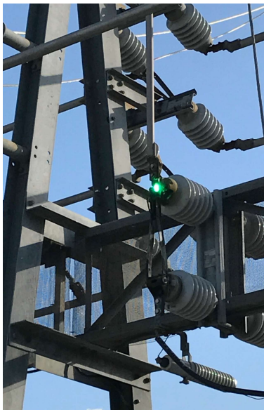
Figure 3: Substation switch identified by DFA
